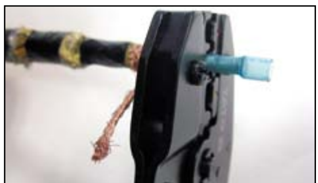
8 Place the connector on the end of the conductor core and crimp it into place.
